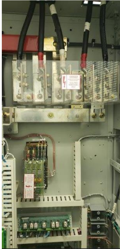
Representative Existing Exciter Hardware
